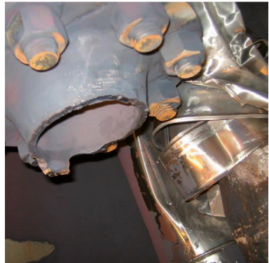
Fig. Broken Inlet Steam Pipe Due to Fatigue in a Position Exposed to High Temperature and a High Stress Level
