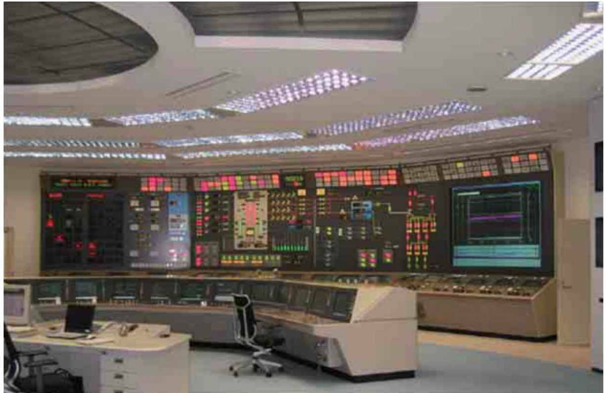
Fig. Main Control Board of NUCAMM-90 for the 1356MW Kashiwazaki- Kariwa Unit 7
