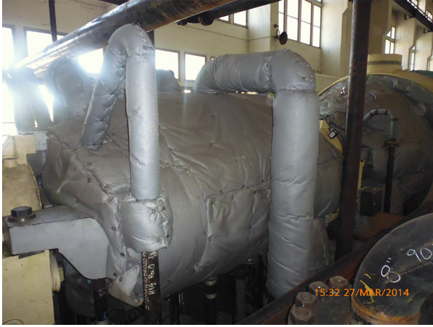
Fig. 2 Thirty megawatt steam turbine unit—photo from power plant
