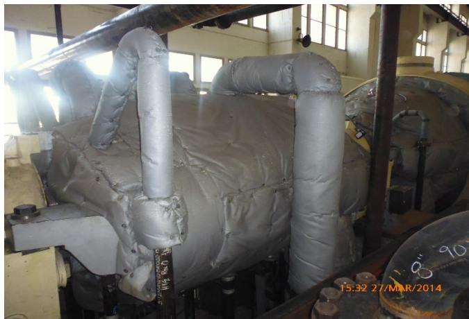
Figure 2: 30MW Steam Turbine Unit – Photo from Power Plant
